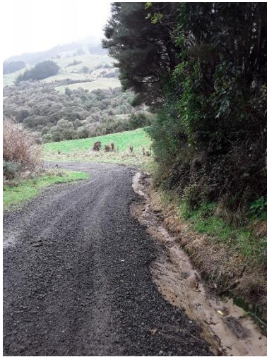
Figure 7: Evidence of rutting within the road surface.
