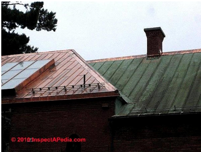
Figure 19. The picture shows a maintained roof and an unmaintained roof with copper cladding. Maintenance would slow the patina layer formation down leading to lower copper concentrations in receiving waters.
