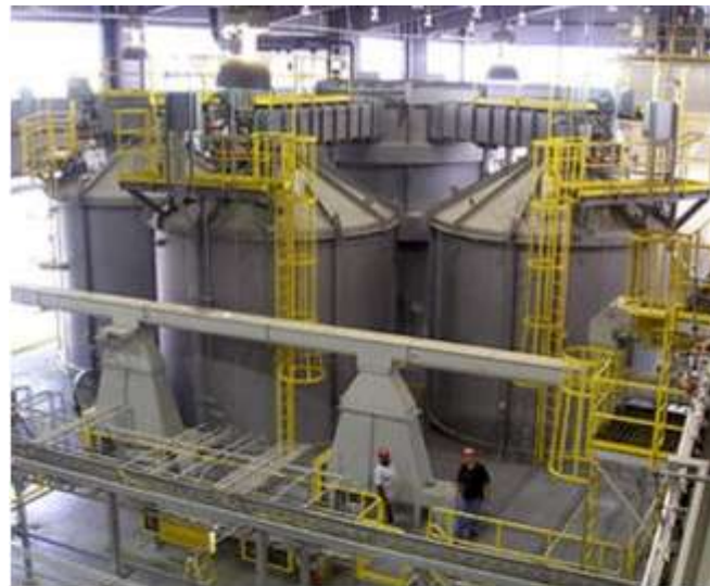
Gasifiers and metering bins at USC plant
